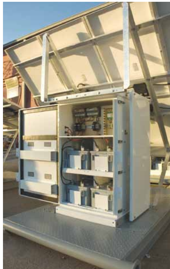
Solar panels mounted to the enclosure produce shade, and additional side sun shade panels create passive cooling to help moderate interior temperatures in battery enclosures. Keeping the battery enclosure cool extends the life of the batteries.
