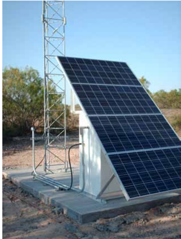
Shading, even small area of the solar panel, greatly decreased power production. This power system will not perform well due to shading from nearby vegetation and improper orientation.
