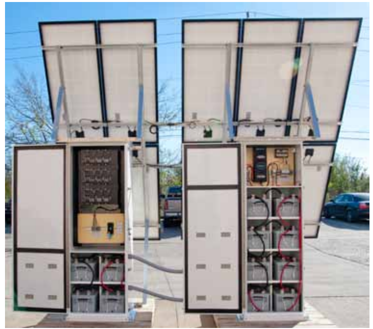
This solar power system for an AC power application required a second enclosure and battery bank to compensate for the power lost in conversion from AC to DC.
