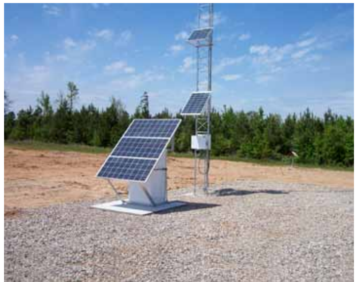
This system is well placed away from obstructions and is oriented to receive maximum solar radiation.
