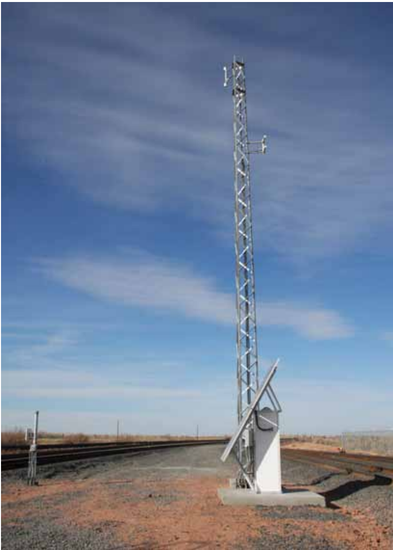
A remote solar power system correctly deployed at a northern location. The array is facing due south, the tower does not cast any shadow on the solar panel, and the panel array tilt angle is correctly calibrated for the latitude less 15°.
