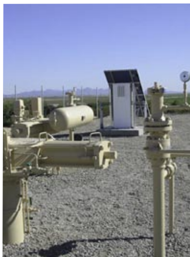
▲ This solar powered block valve on a pipeline in the Imperial Desert is a good example of a critical load; failure to operate properly can result in an environmental disaster.
