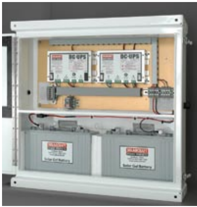
▲ This high reliability DC-UPS system for a refinery features redundant power supplies, each capable of running the load by itself.
