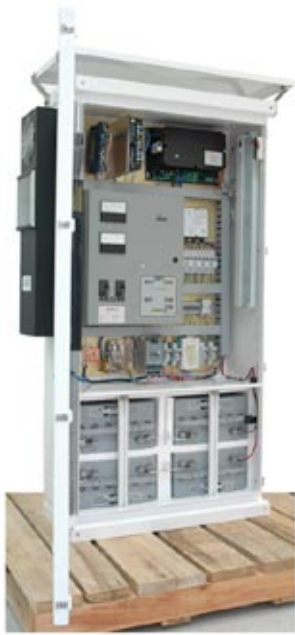
▲ This DC UPS system for a Texas electrical substation utilizes a high reflectance finish, sun shade and air to air heat exchanger to keep internal temperatures down. Note the heavy duty shipping pallet -cheap insurance to prevent damage in transit.
