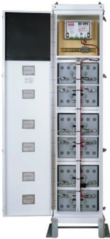
▲ When sizing and designing a high reliability system, always consider the consequences of failure. This small footprint UPS offers 21 days of autonomy (battery reserve) for an offshore platform, long enough to ride out a hurricane.
