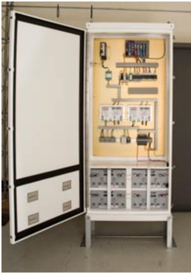
▲ This well integrated system includes the DC-UPS power supplies, power distribution circuit breakers, batteries, surge protection, RTU with interface electronics and communications. This single enclosure replaced four separate enclosures and a rack, resulting in considerable savings in both equipment costs and installation time.
