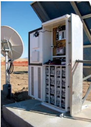
▲ A well engineered solar system will provide years of reliable, trouble free service in all weather conditions.
