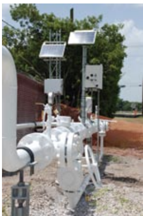
▲ Systems rated for hazardous locations, such as pipeline meter stations, must be certified as a complete system, including the loads and external conduit and cabling.
