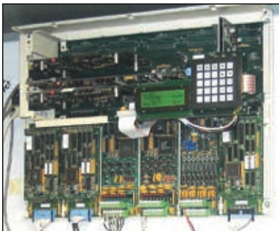
▲ Typical Bristol 3330 installation.
