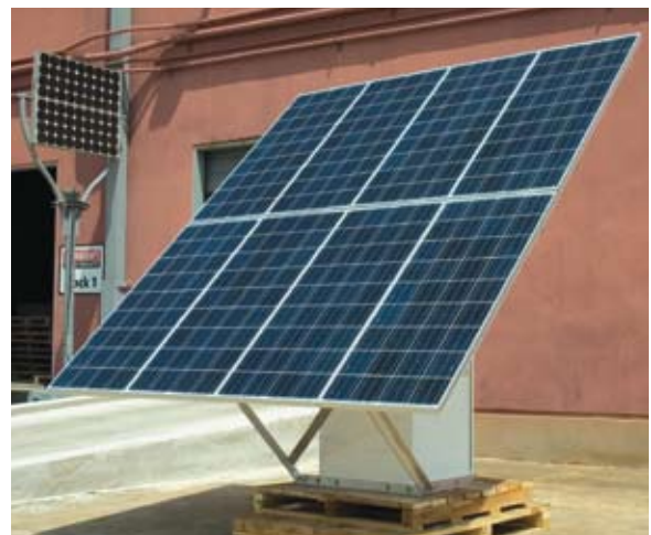
▼ 1KW unitized system utilizes the large array for enclosure shading
