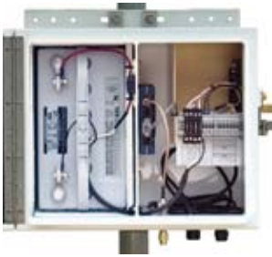
▲ Solar powered single battery configuration: 110Ah battery, 40W or 50W solar panel, solar controller, load terminal for flow computer, and radio.
