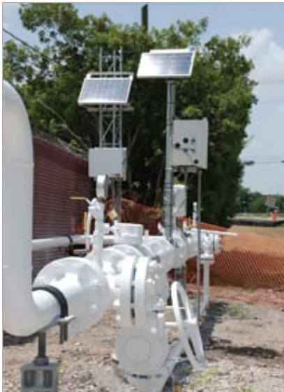
▲ Solaradio (pictured on the left) transmits information from a TotalFlow computer at a custody transfer station
