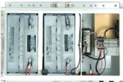
▲ Solar powered two battery configuration: two 110Ah batteries, 85W solar panel, solar controller, load terminal for flow computer, and radio.
