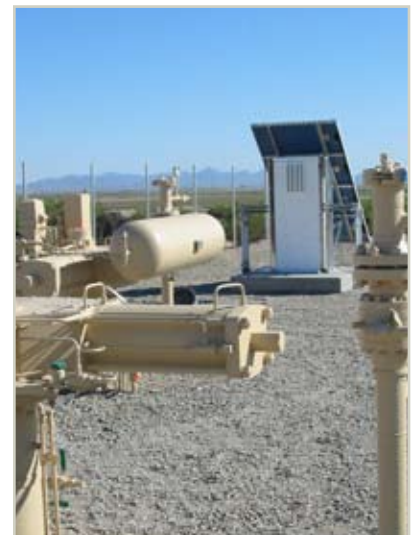
▲ Double-wide Uni-Pak™ deployed for pipeline control of block valves, Mohave Desert.
